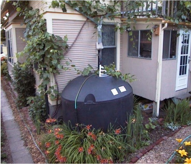
RAINWATER COLLECTION SYSTEM AT A PORTLAND, OR HOME
